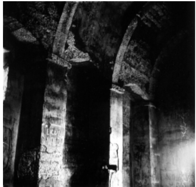
Crkva Sv. Mikule u Dobrovi kod Labina, pojasnice svoda (foto: Državna uprava za zaštitu spomenika kulture i prirode, Rijeka) Church of Saint Nicholas in Dobrova near Labin, reinforced vaults (photo: The State Office for the Protection of the Cultural and Natural Heritage, Rijeka)
